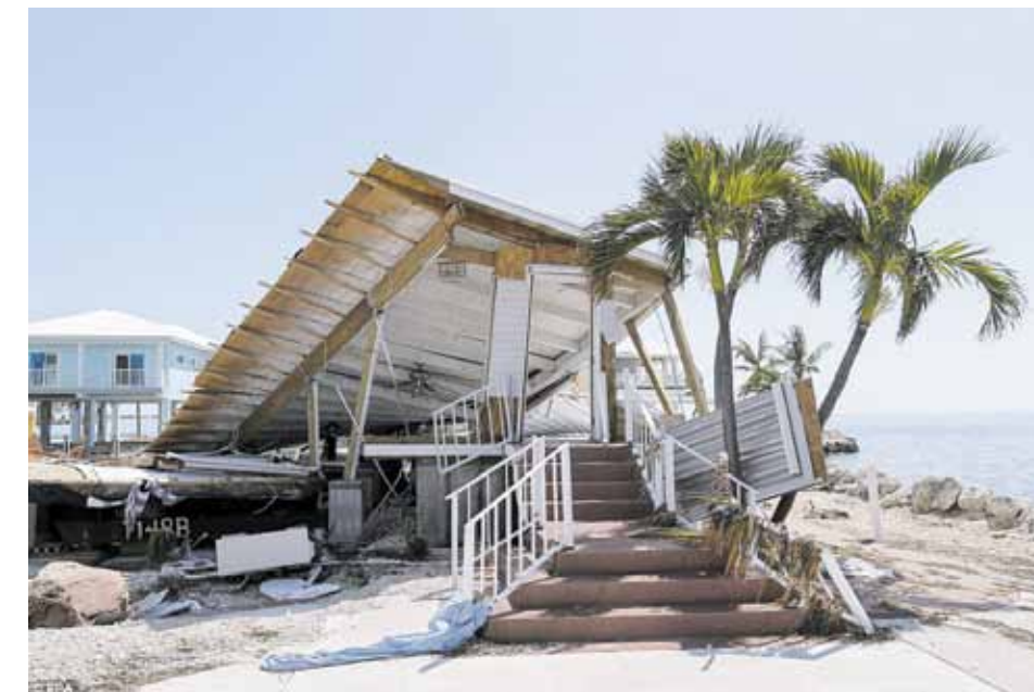
It must have been a shock when the owners of this Marathon home returned.
