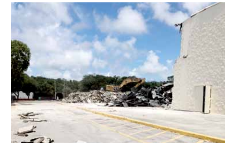
Demolition of Kmart, preparing space for the new Publix in Key Largo.
