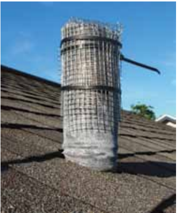
Cover roof vent pipes with hardware cloth and wire mesh to prevent entry into buildings by Cuban Tree Frogs. Credit: UF/IFAS
